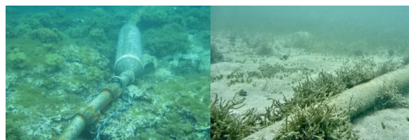
Fig. 1. Photographs of underwater electrical cables.
