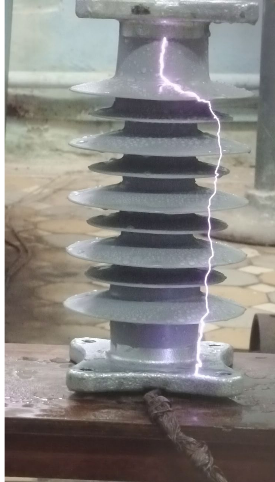
Fig. 9. Overlapping of the moistened insulator.
